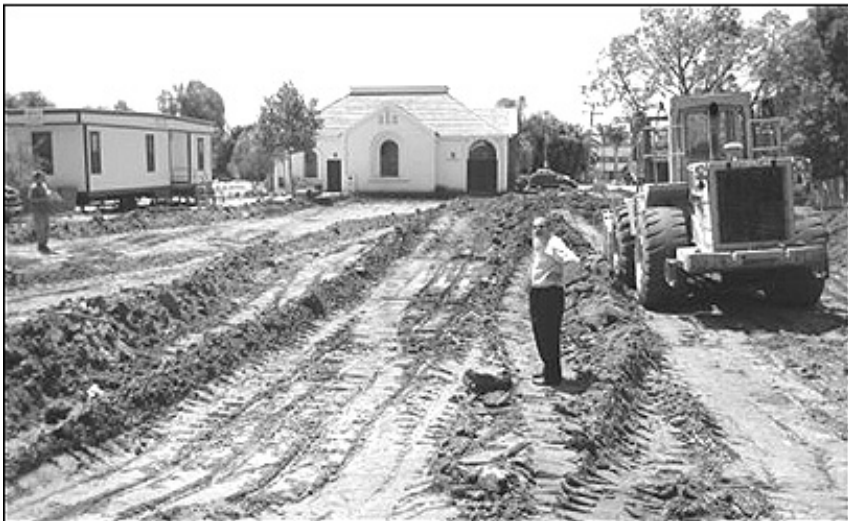
Rabbi Eliezrie surveying the lot during grading, prior to excavation for the foundations of the new building.
